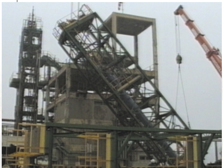
Placement of a 50 t/d 100% HCl skid
